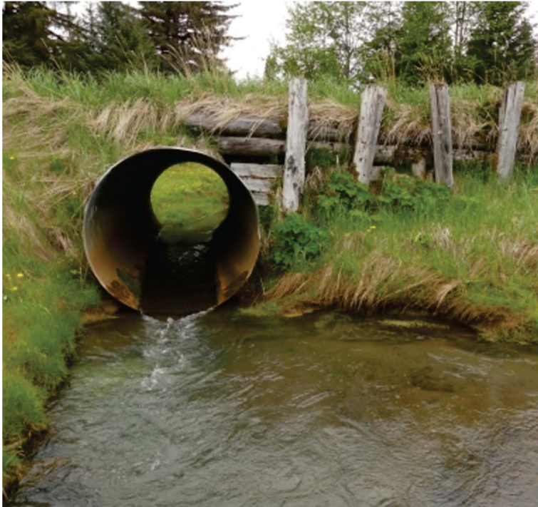
A perched culvert that's undersized passes Harry Hall Creek under a road in Gustavas, Alaska.
