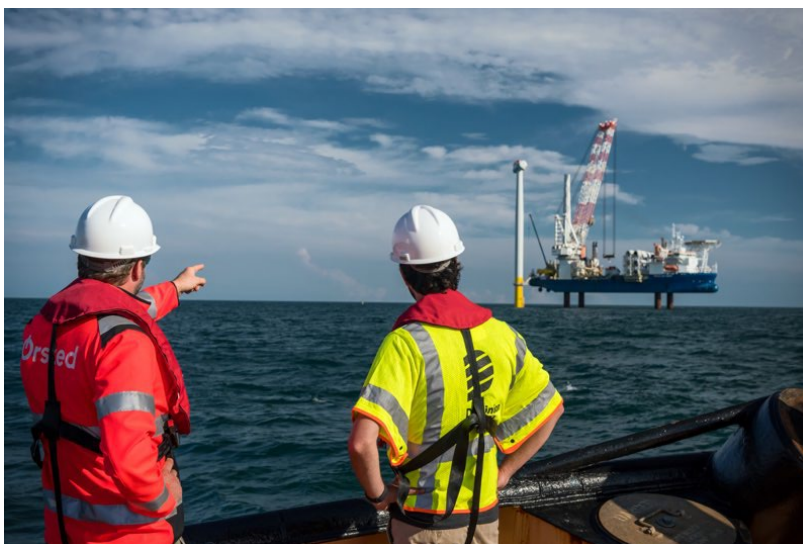
TWO EMPLOYEES WATCHING OFFSHORE WIND TURBINE INSTALLATION (SOURCE: BSEE RENEWABLE ENERGY PROGRAM)
