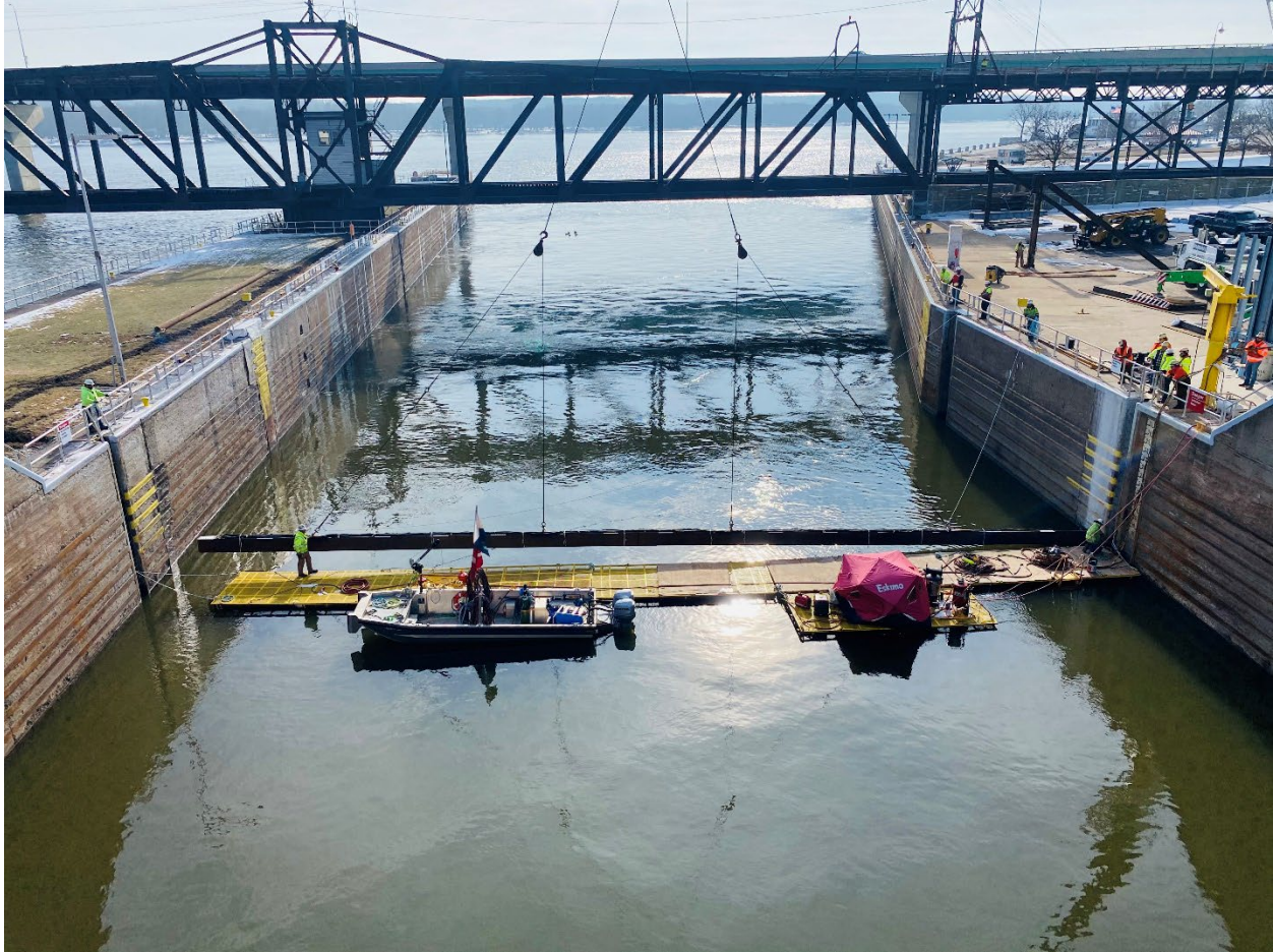
THE UADS SOUNDBAR, COMPRISING 16 UNDERWATER SPEAKERS AND SCIENTIFIC MONITORING EQUIPMENT, WAS INSTALLED IN THE LOWER LOCK APPROACH CHANNEL OF LOCK 19 ON THE UPPER MISSISSIPPI RIVER IN KEOKUK, IA, IN FEBRUARY 2021 (SOURCE: USGS)
