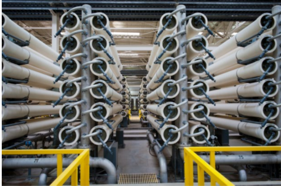
TUBULAR MEMBRANES AT RECLAMATION'S YUMA DESALTING PLANT IN YUMA, ARIZONA (SOURCE: BUREAU OF RECLAMATION)
