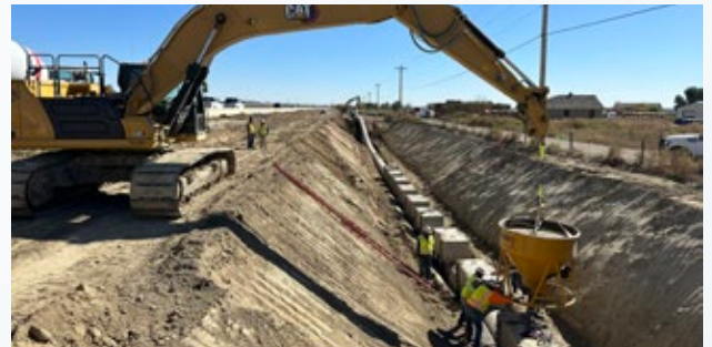
Construction of the first segment of the trunkline of the Arkansas Valley Conduit in 2023. Current phases of the project are utilizing BIL funding to bring clean and reliable water supplies to communities east of Pueblo, Colorado. Reclamation Photo.
