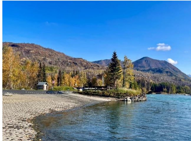
Kenai NWR – Replacement Boat Launch, Parking Improvements and Public Restrooms at Jim's Landing. Credit: PND Engineers, Inc
