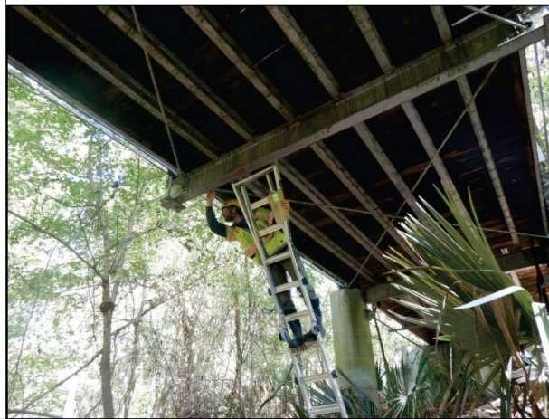
Hands-On Inspection of NSTM of the Iron Bridge at Tensas River National Wildlife Refuge, Louisiana
