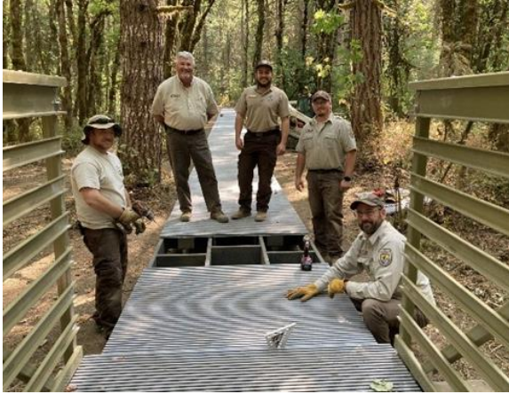
GAOA MAT Strikeforce Team Members Constructing a Replacement Accessible Trail Bridge at the William I. Finley NWR. Credit: USFWS
