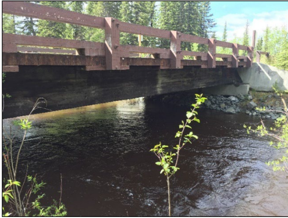
Before photo of timber bridge at Sourdough Campground. Photo Credit: Curt Fortenberry
