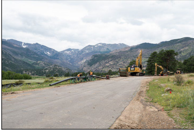
Fusing HPDE pipe for installation in front of Moraine Park Meadow and the divide. Photo Credit: Jamie Richards
