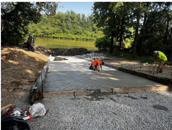
Construction on a boat launch at Dale Bumpers White River National Wildlife Refuge. Photo Credit: USFWS
