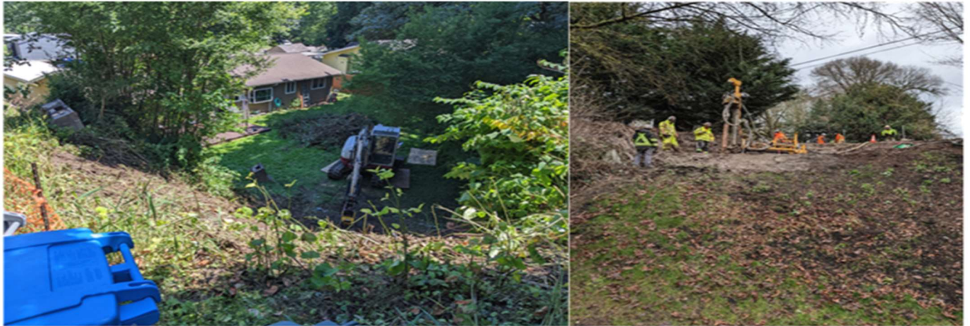
Photo on left: looking down from the access road to the community into the private property, showing the excavation of the subsidence feature and construction of the slope toe buttress to stabilize the slope. Photo on right: the drilling and grouting of the mine tunnel entry and underground mine voids in the slope soils above the subsidence feature. Photos taken by Cody Yankey, OSMRE Project Manager on 6/27/2022 (before) and 3/3/2023 (work in progress).
