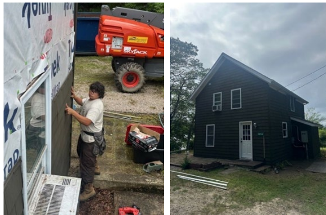
GAOA Funded Maintenance Professional Replacing Siding on a Quarters building at Ninigret NWR. Image: USFWS
