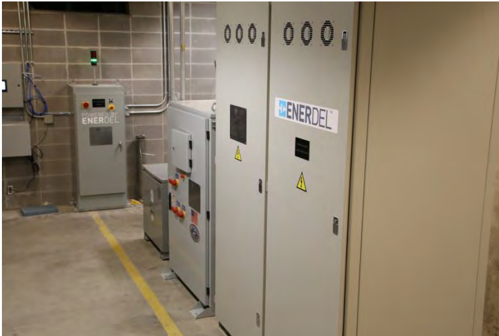
Figure 4-3 Lithium Ion Battery Energy Storage System Located at the Black & Veatch Headquarters
