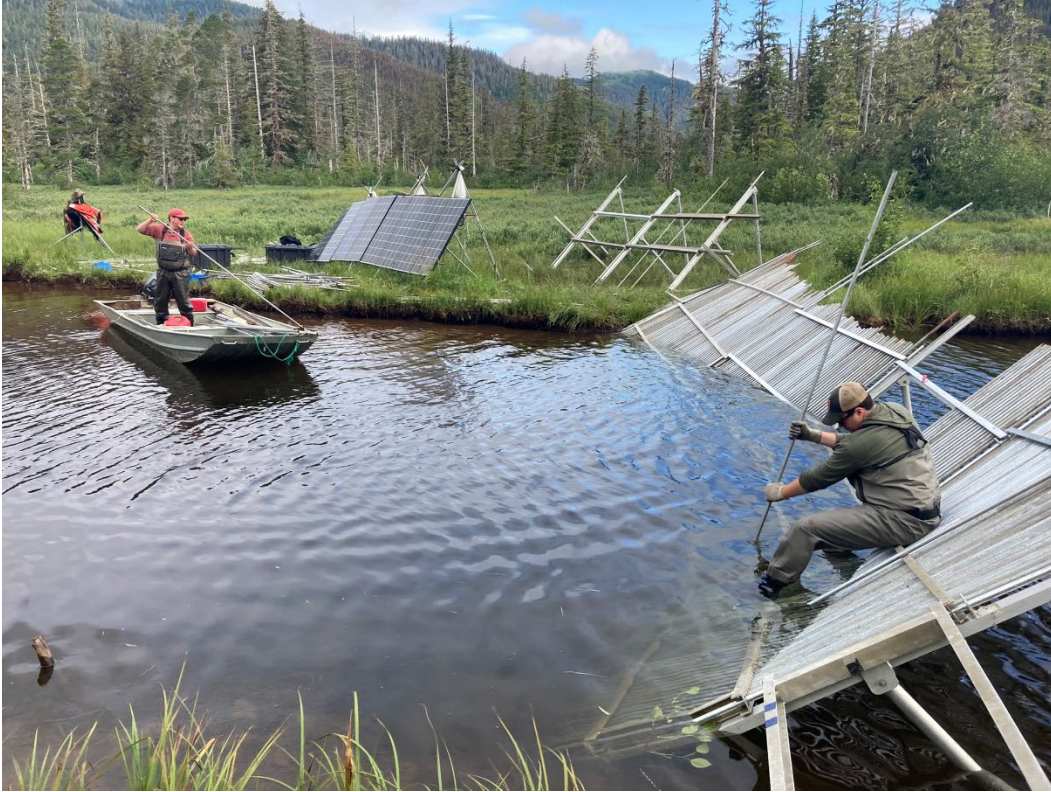
Figure 1. Matt Swift (left, in boat) and Taylor Cunningham installing the Sitkoh Lake weir, July 14, 2022.
