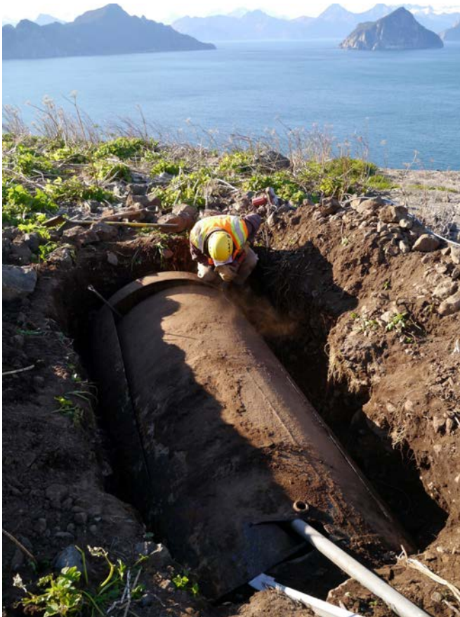
Removal of an underground storage tank on Barwell Island in the Alaska Maritime NWR, AK.
