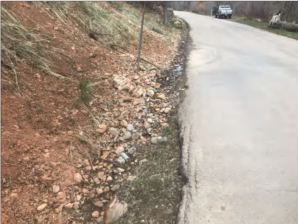
**Mile marker 1.1 furthest downstream visible H. sulfide input into Upper Diamond Fork.
