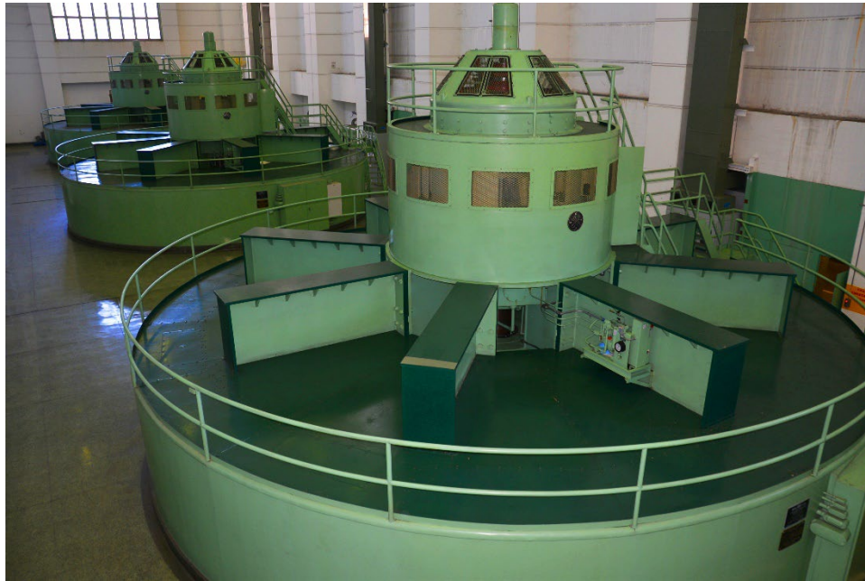
HYDROPOWER TURBINES AT KESWICK POWER PLANT NEAR REDDING, CA. RECLAMATION FACILITIES PROVIDE HYDROPOWER FOR MILLIONS OF U.S. HOUSEHOLDS, AND ITS RESEARCH AND DEVELOPMENT WORK FINDS SOLUTIONS TO KEEP BOTH WATER AND POWER FLOWING. CREDIT: BUREAU OF RECLAMATION
