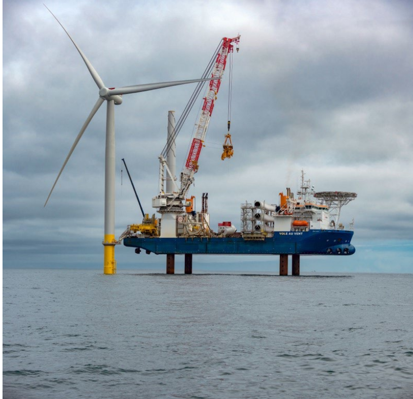
CRANE INSTALLING AN OFFSHORE WIND TURBINE. BSEE IS COLLABORATING WITH ACADEMIA, INDUSTRY, SCIENTISTS, AND OTHER GOVERNMENT AGENCIES TO CONDUCT RESEARCH THAT MAKES OFFSHORE ENERGY PRODUCTION SAFER. SOURCE: BSEE
