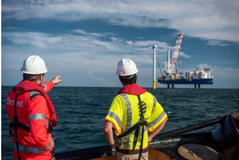
TWO EMPLOYEES WATCHING OFFSHORE WIND TURBINE INSTALLATION. BSEE IS RESEARCHING OPTIONS FOR REMOTE INSPECTIONS, WHICH COULD ENSURE SAFETY MORE EASILY THAN DIRECT INSPECTIONS. SOURCE: BSEE RENEWABLE ENERGY PROGRAM
