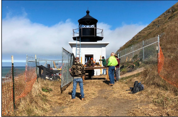
Workers completing structural renovations on the Punta Gorda Lighthouse, Photo Credit: BLM, B. Donaldson
