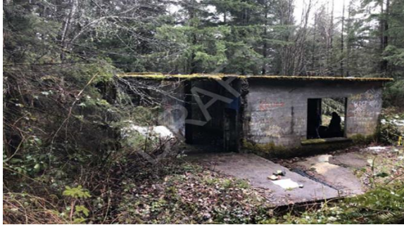
WA-21-002 Project: Hazardous facility with temporary steel plate restricting access to vertical opening
