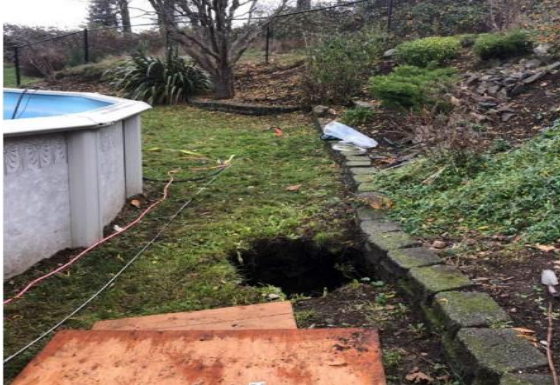
WA-21-005 Project: Vertical opening between swimming pool and retaining wall.
