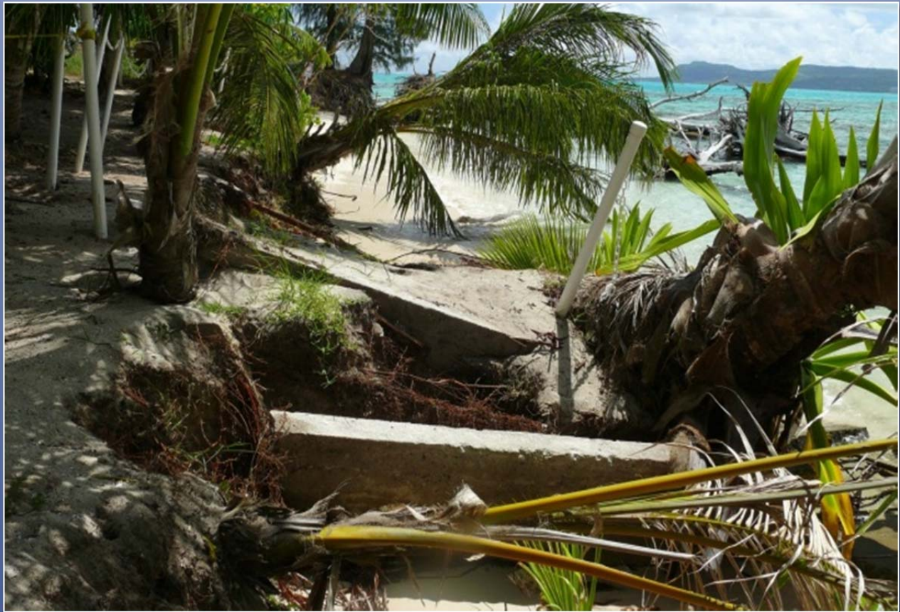
Shoreline erosion, Managaha Island, Northern Mariana Islands
