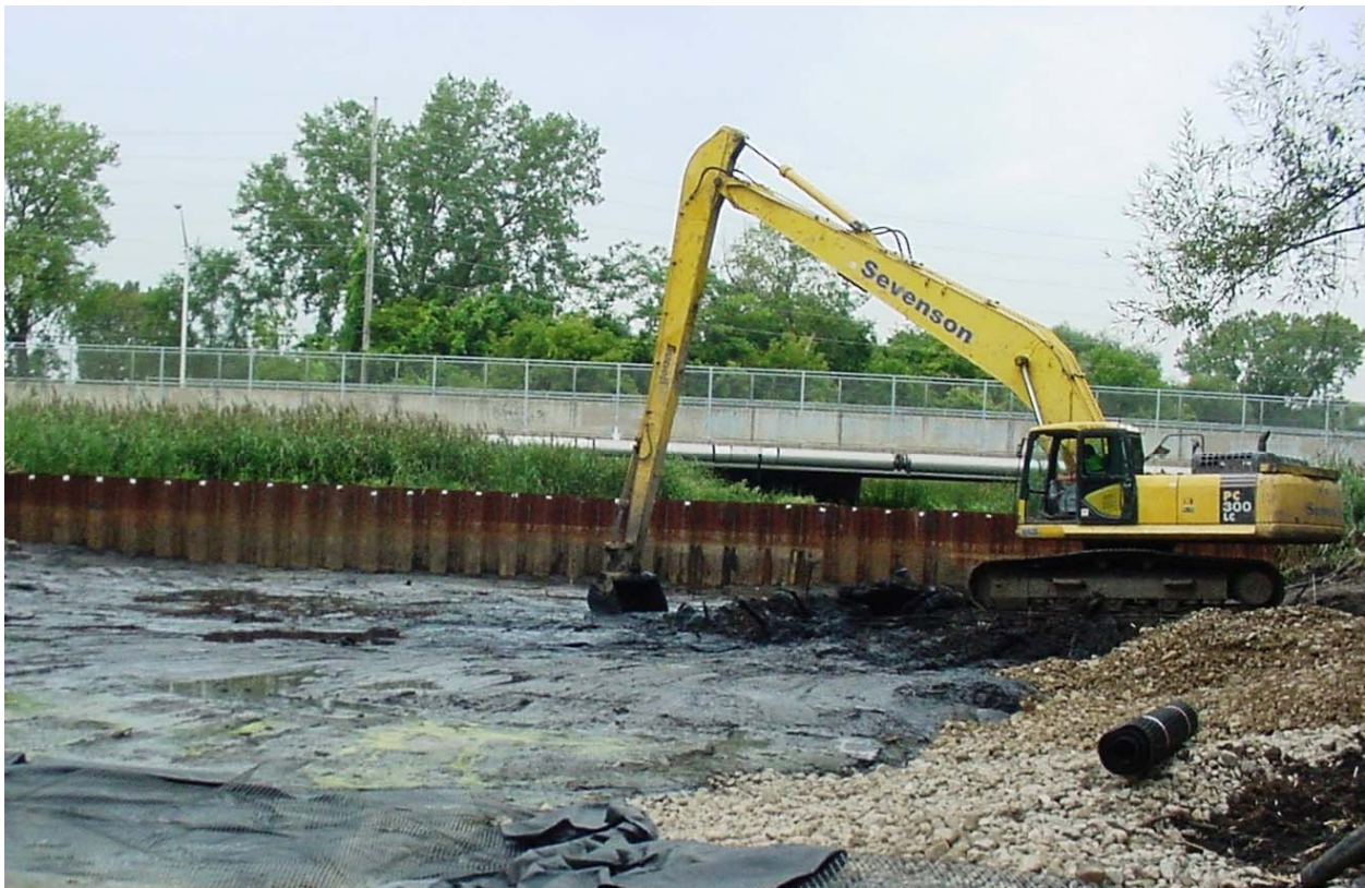
Contaminated sediment removal – the first phase of Grand Calumet River, IN stream restoration. (FWS photo)
