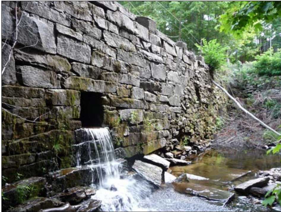
Figure 4. Downstream face of the Bartlett Rod Shop Company dam with mid-level outlet, releasing Amethyst Brook flows.
