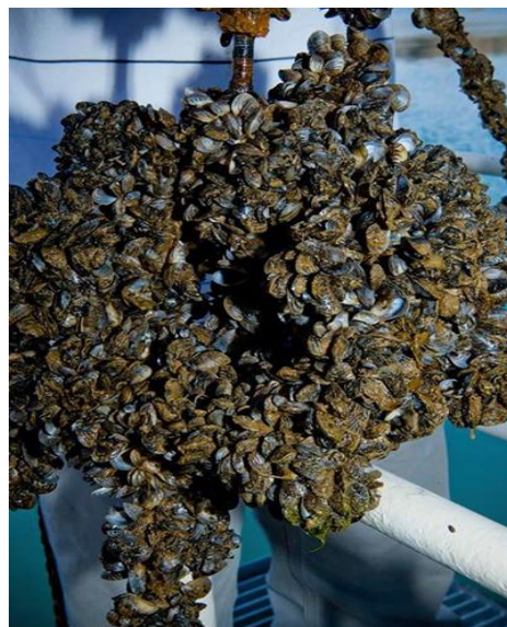
Reclamation has pioneered new methods to aid early detection of quagga and zebra mussels before they become a major nuisance for water infrastructure.
