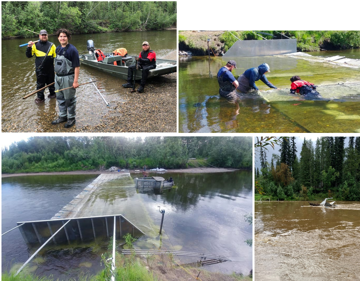
Clockwise from top left: TCC fisheries technicians Spencer Jacobs, Nick Jacuk, and Robert Rowe and ANSEP student intern Archer Bowles, Henshaw crew building weir, flash flood submerged weir and debris destroyed sampling cage, completed weir build June 2021.
