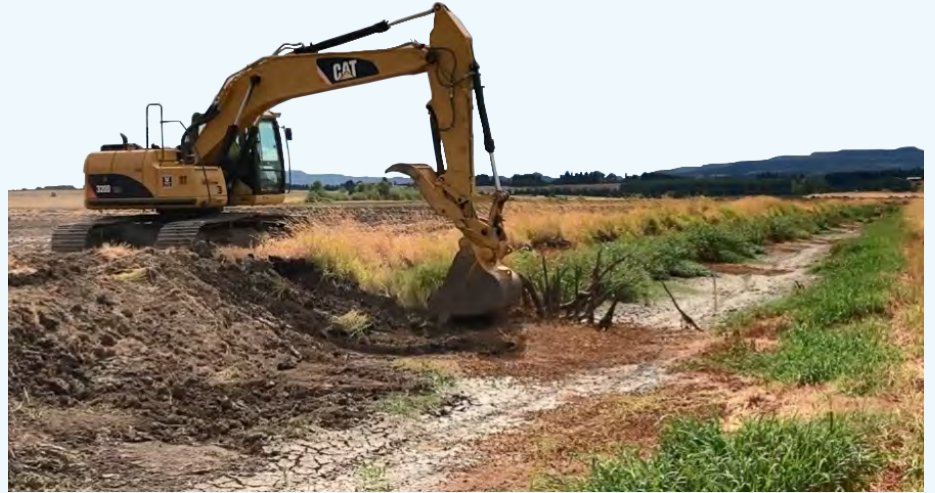
Heavy machinery operated by MAT staff was used to dig a new stream channel and place large woody debris to provide forage and protected areas. Photo credit: Graham Evans-Peters, USFWS
