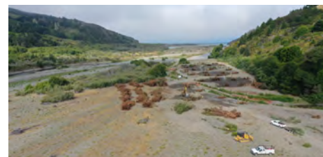
Willow and large wood structures were strategically installed to provide roughness in the channel and promote the formation of diverse habitats. Photo credit: Hugh McGee
