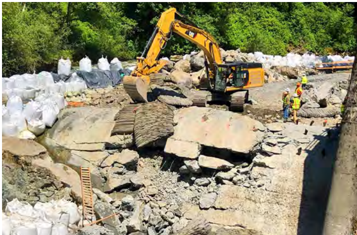
Removal of the Middle Fork Dam on the Nooksack River. Photo credit: City of Bellingham, Washington.
