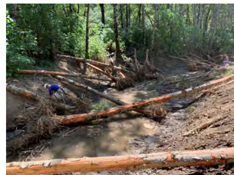
A restoration worker installs wetland plants in the newly excavated slough channel. Photo credit: Hugh McGee
