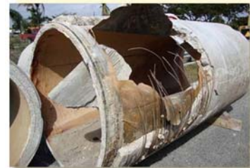
Failed PCCP in Miami, FL
