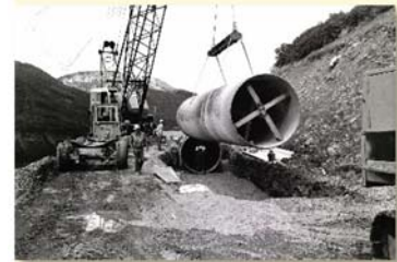
Contractor laying a 40-ft section of the North Fork Pipeline during the original construction
