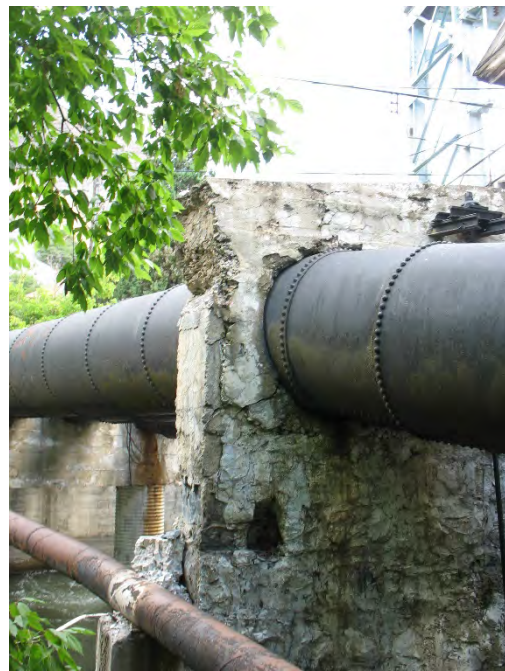
Concrete deterioration on penstock supports
