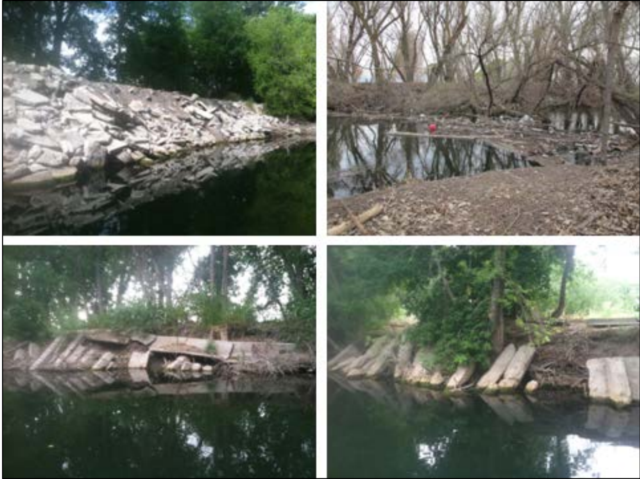
Figure 3-27. Steep banks covered in concrete and trash accumulations are common along the existing river channel. The top left photo shows the existing steep concrete covered south bank just downstream of the Utah Division of Wildlife Resources fish weir. The top right photo shows trash and organic debris accumulations in the existing channel. The bottom photos show the trail and steep concrete covered northern bank downstream of Alligator Park.
