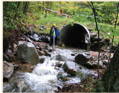
◀A recently installed arched culvert designed with the Stream Simulation Approach on the Green Mountain National Forest days after the Hurricane Irene catastrophe shows no stream blockage. USDA Forest Service photo.
