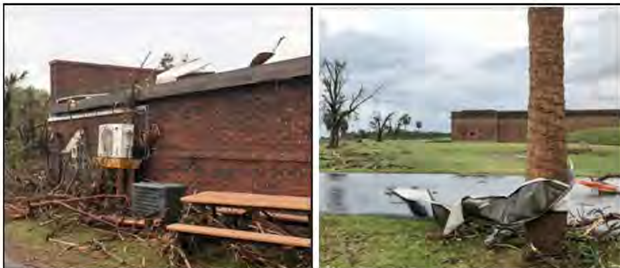
NPS Damage Images
