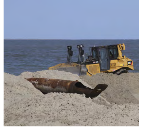
Beach renourishment activities at Wallops Island, VA, part of the barrier islands that stretch along the eastern seaboard of the United States. Photo credit: Patrick Bloodgood, USACE
