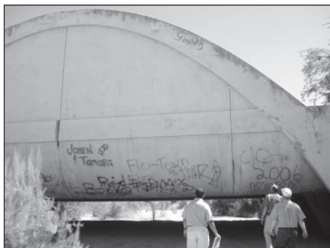
Deteriorating China Wash Flume
