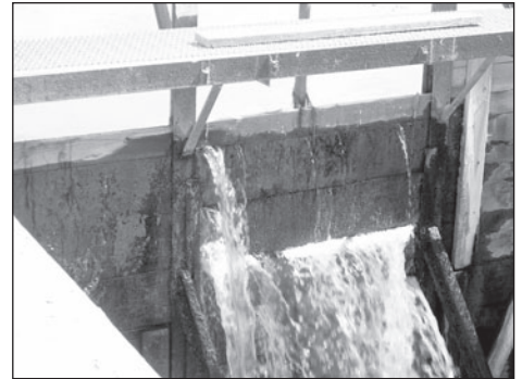
Leaking Check Gate
