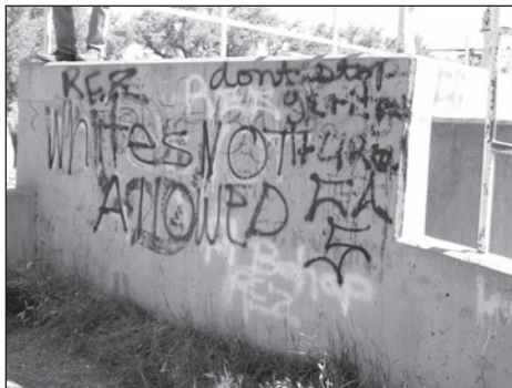
Source: GAO. Graffiti on Irrigation Structure
