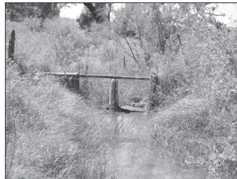
Overgrown Vegetation Around Dilapidated Irrigation Check Structure
