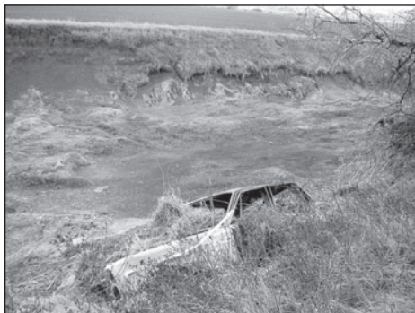
Source: GAO. Abandoned Car in Deteriorated Canal
