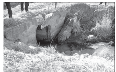
Crumbling Concrete Structure
