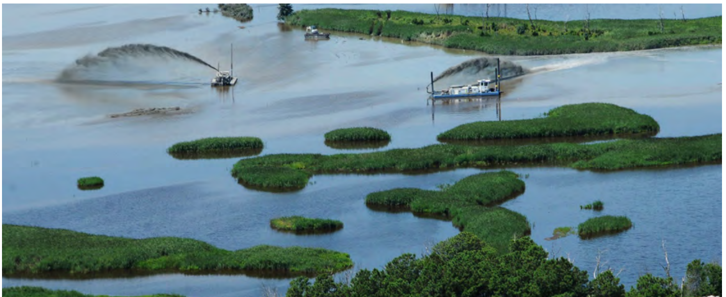
Dredges working to create channels to restore tidal flow in the back bay marsh areas of the Prime Hook Refuge. Photo credit: USFWS
