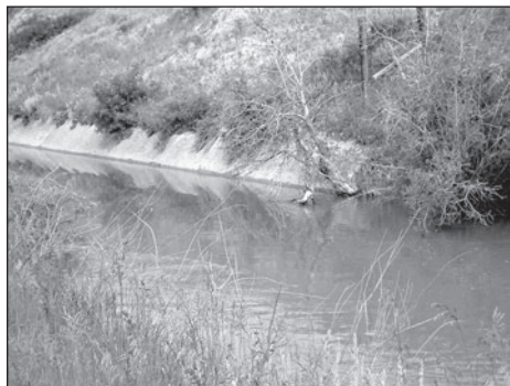
Source: GAO. Deteriorating Canal Lining
