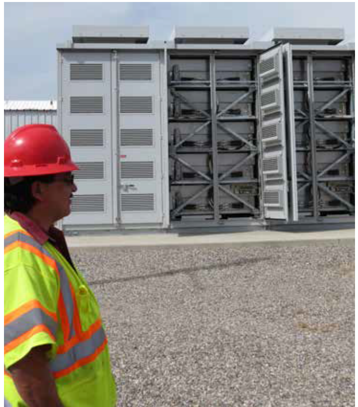
Energy Storage pilot project in Los Alamos County. Photo Credit: Ken Hughes
