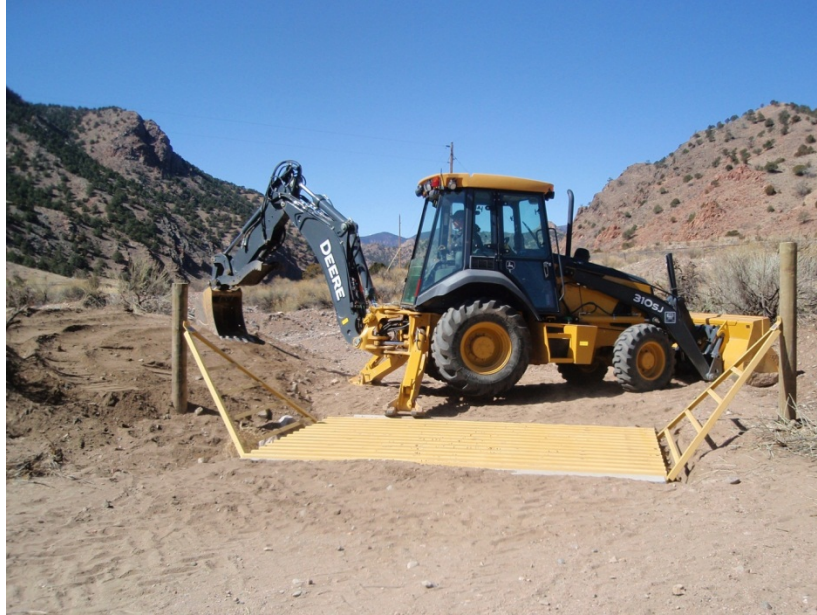
Installation of a cattleguard, in cooperation with the Colorado Parks and Wildlife, is used to provide access to the Arkansas Headwaters Recreation Area and prevent livestock from getting out onto the highway.
