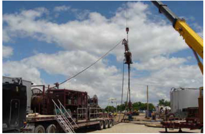
Specialized drilling equipment being used to re-enter the I&W brine cavern in Carlsbad.
