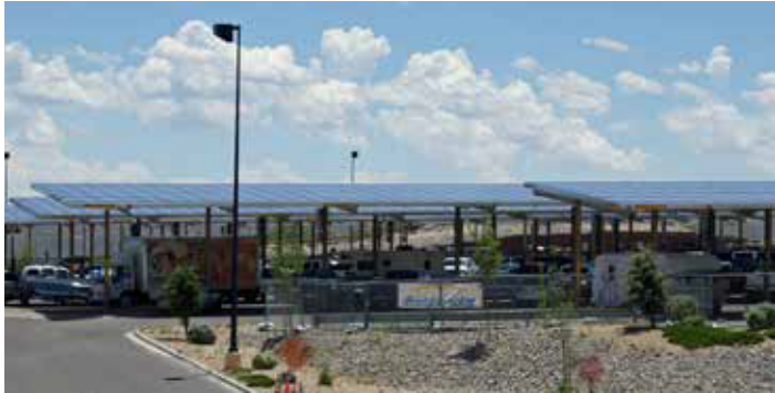
1 MW Solar Power Parking Lot at the Walmart Parking Lot in Truth or Consequences (Photo Credit: M. Gaiser)
