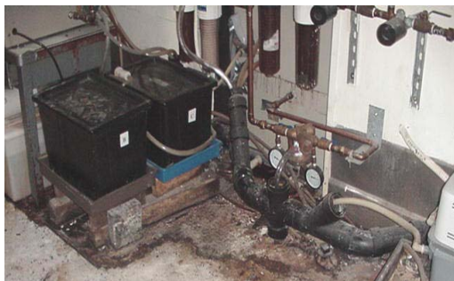
Tropic Humidity and deterioration
