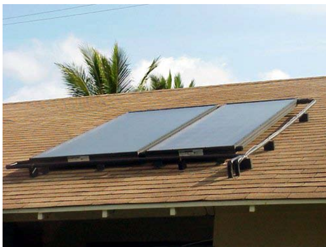
Figure 20. Residential Solar Hot Water, Hickam AFB, Hawaii
