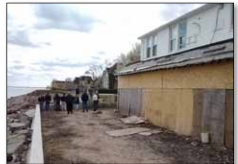
The south shore of Staten Island was hit hard by Hurricane Sandy in 2012, and the damage is still apparent in some areas. Photo credit: Jeff Danielson, USGS.
