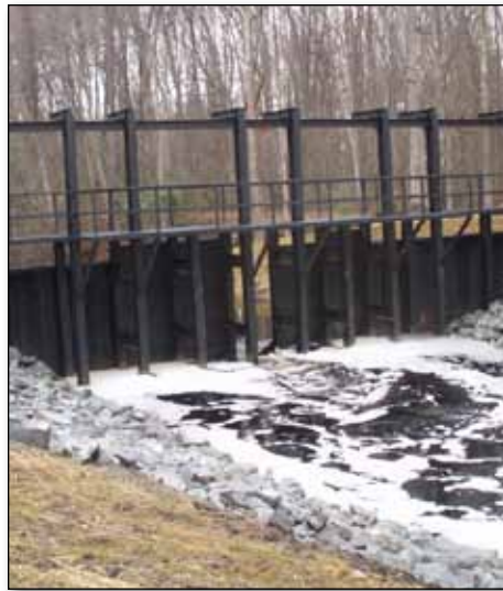
Above- A new water control structure on the South Martha Washington Ditch in the Dismal Swamp State Park. This new weir restored critical hydrologic features within the Great Dismal Swamp.
