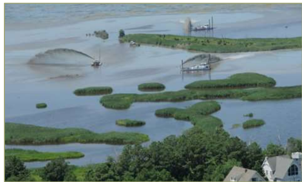
Dredge work to drain flooded marsh at Prime Hook National Wildlife Refuge (Richard Weiner)
