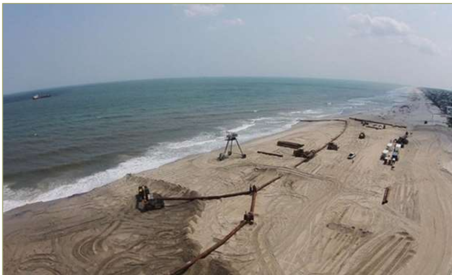
Long Beach Island Coastal Storm Damage Reduction Project, New Jersey (Tim Boyle)
