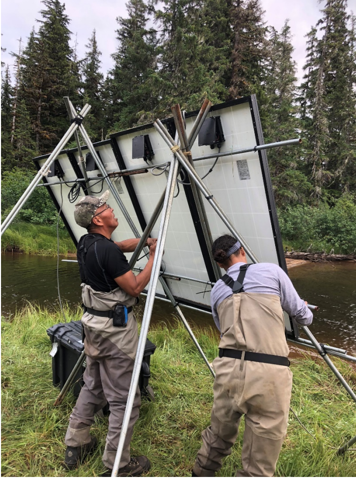
Figure 1. Roger Williams (left, Angoon Community Association) and Amber Wendler (right, Student Conservation Association) install solar panels at the Sitkoh Lake video weir.
