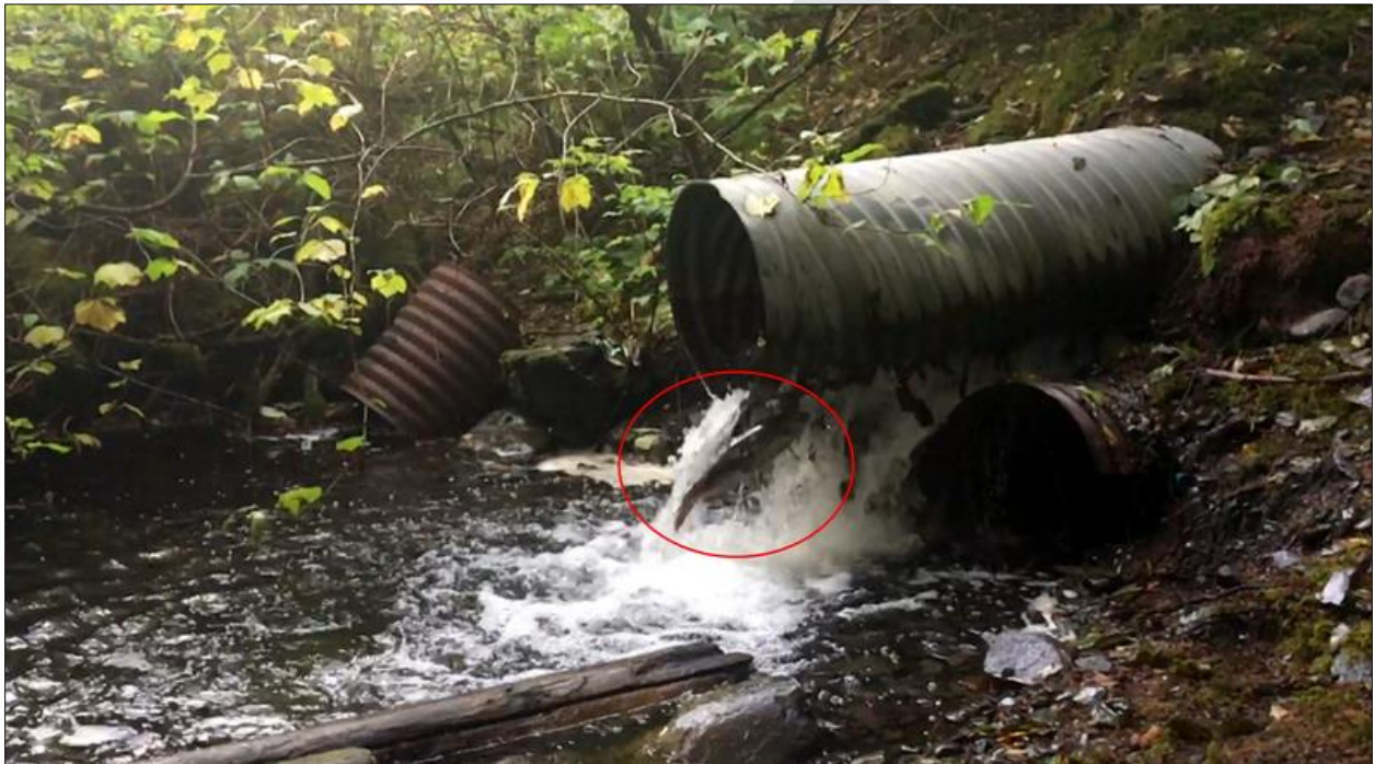
Figure 3. Salmon passage barrier scheduled for replacement at the outlet of Boy Scout Lake. Note the failed attempt of the encircled coho salmon to access the lake via the bottom-corroded culvert. Photo: Franklin Dekker/USFWS.
