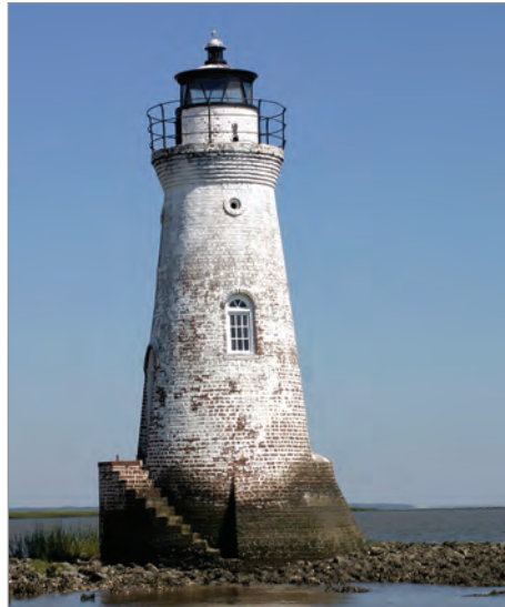
The Cockspar Lighthouse at Fort Pulaski National Monument needs to be stabilized for expected sea-level rise impacts. Photo credit: Paul Brennan
