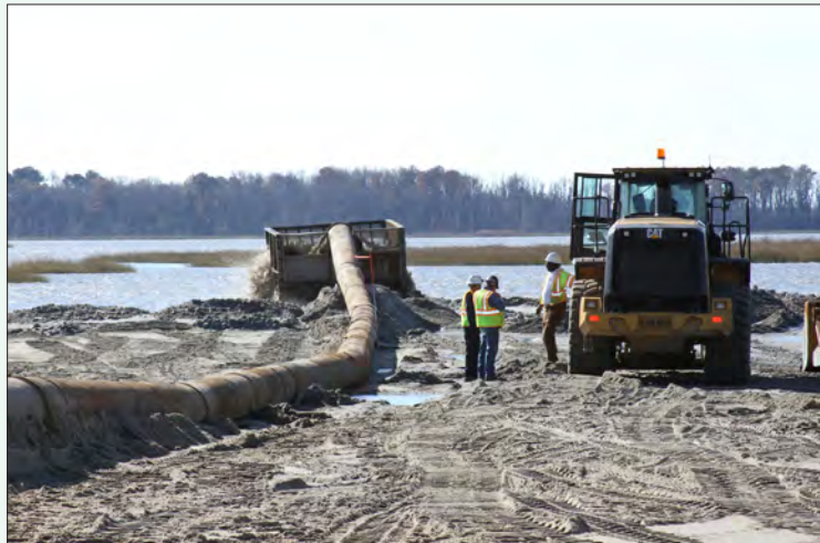
Pumping sand operations to restore beach, dunes and close breaches at the Prime Hook Refuge. Photo credit: Tim Boyle, USACE
