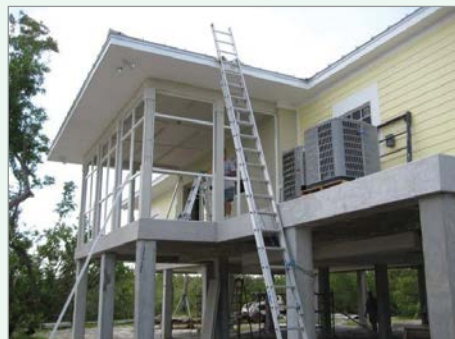
Employee residences on J.N. "Ding" Darling NWR on Sanibel Island, FL, were rebuilt to withstand storm surge and severe storms. Photo credit: USFWS
