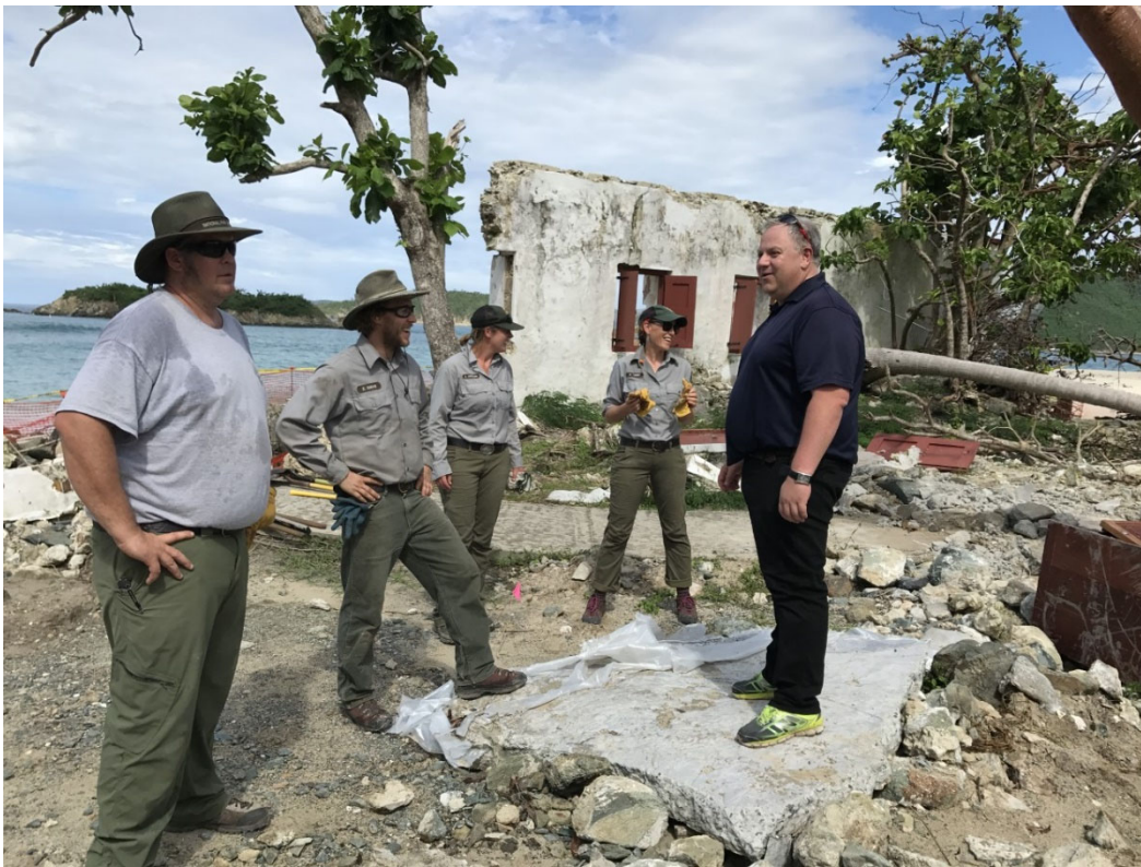
Secretary David Bernhardt inspecting damage with the National Park Service Staff in St. John, USVI, after Hurricanes Irma and Maria
