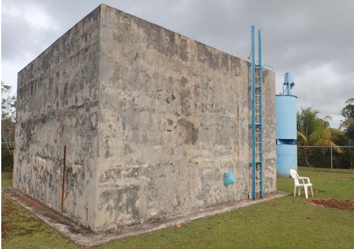
Figure 7.—The concrete disinfection clearwell at Ngardmau plant.
