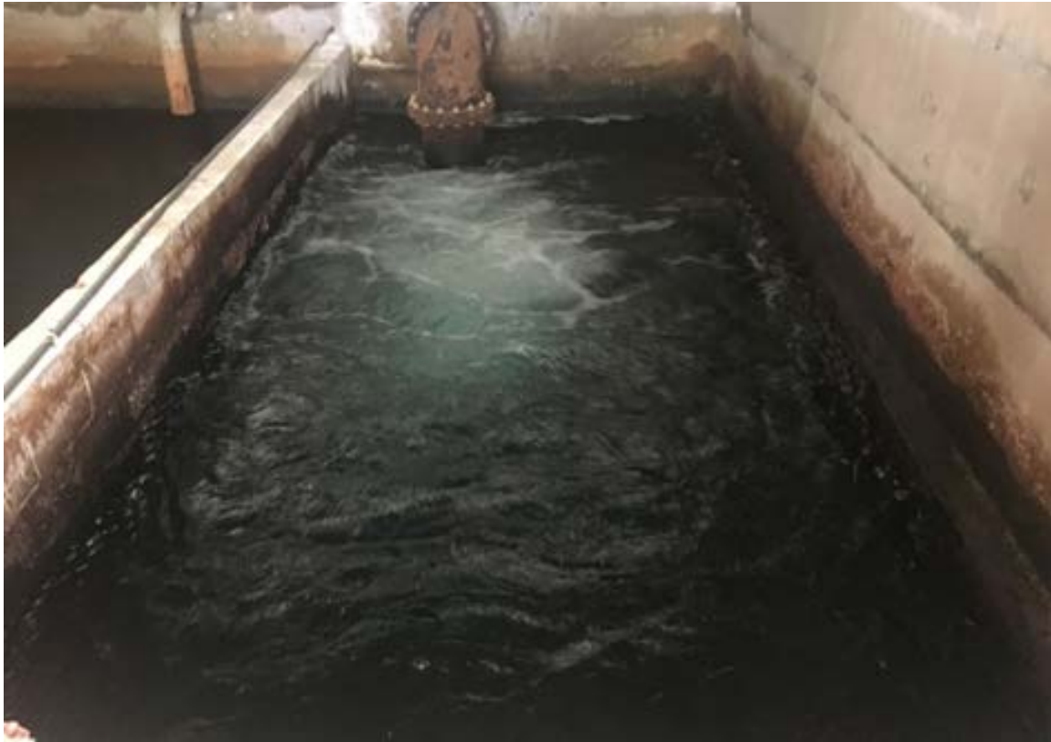
Figure 15.—The inlet basin of the Airai plant clearwell.
