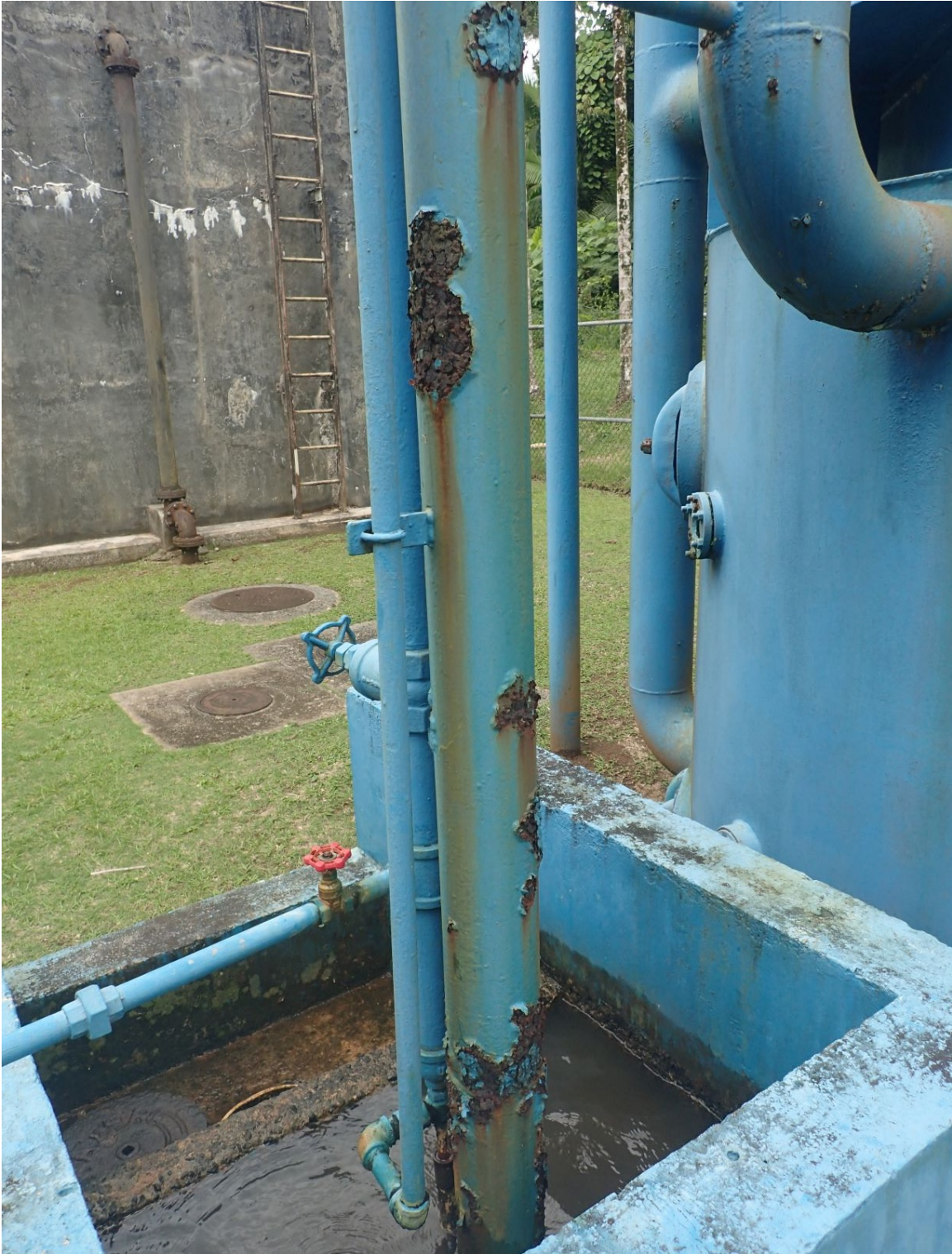
Figure 10.—Corrosion of the backwash pipe on the Ngatpang Mechebechubel filter tank.
