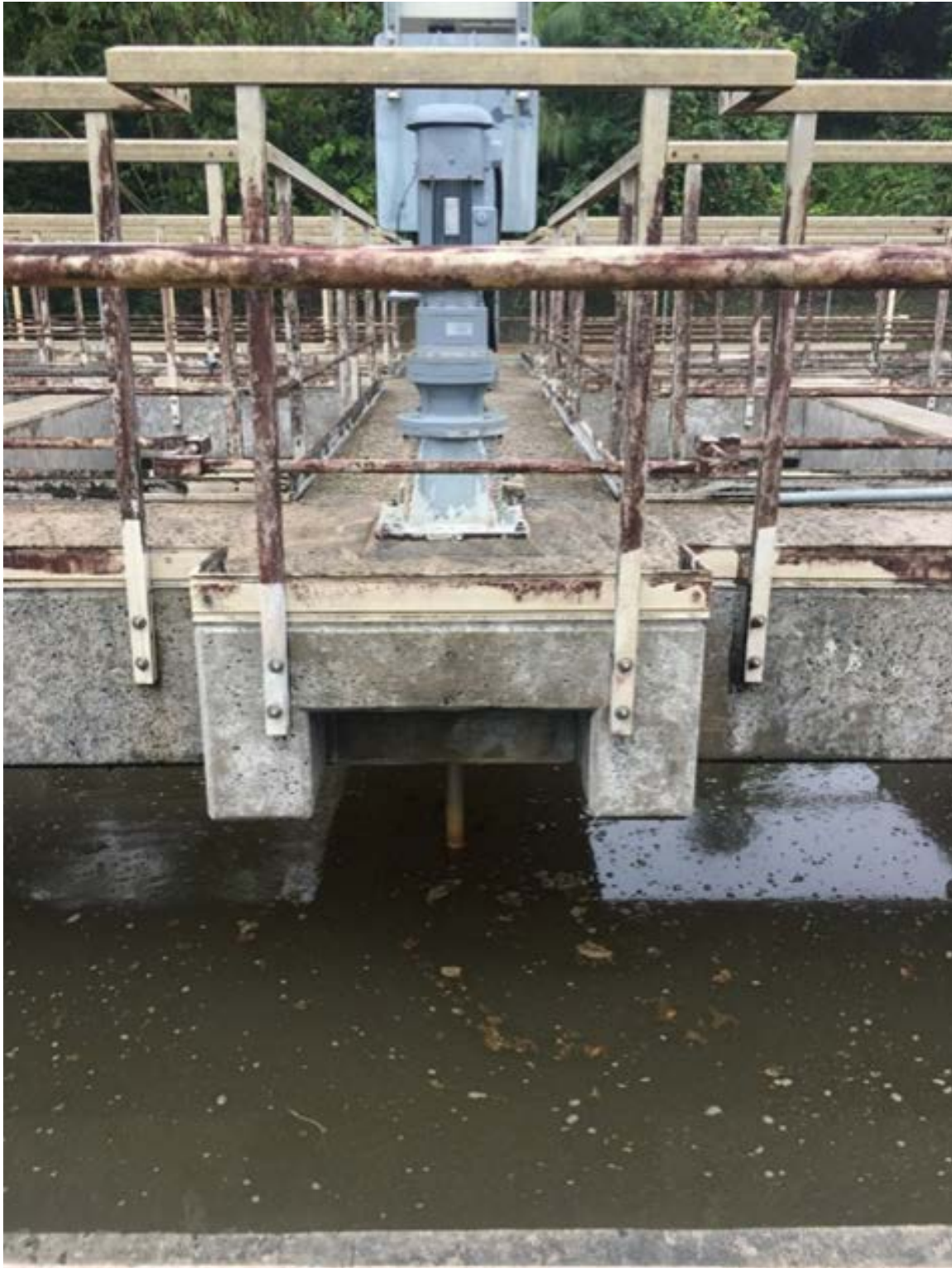
Figure 12.—Flocculation chamber at the Airai plant.
