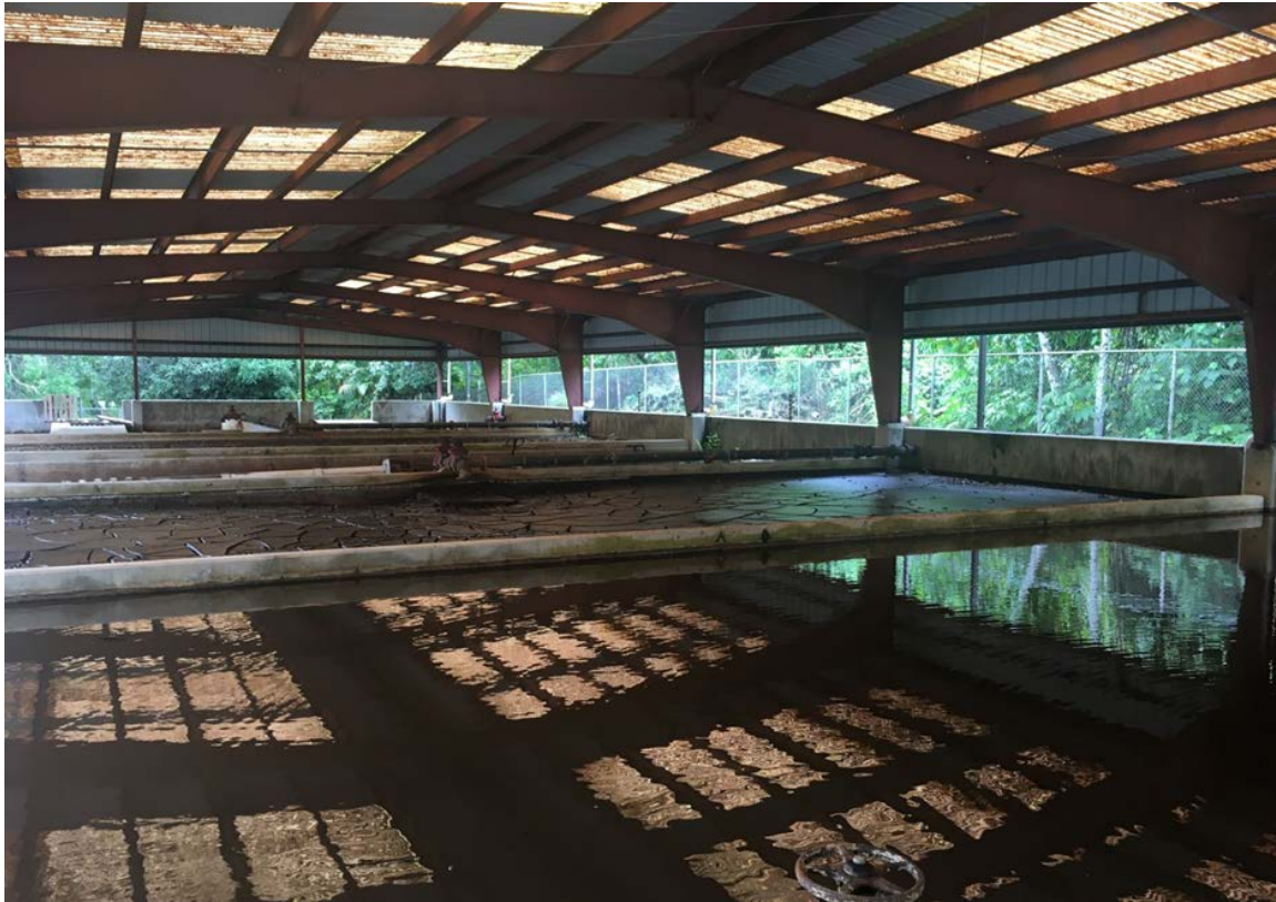
Figure 13.—The sludge drying beds at the Airai plant.
