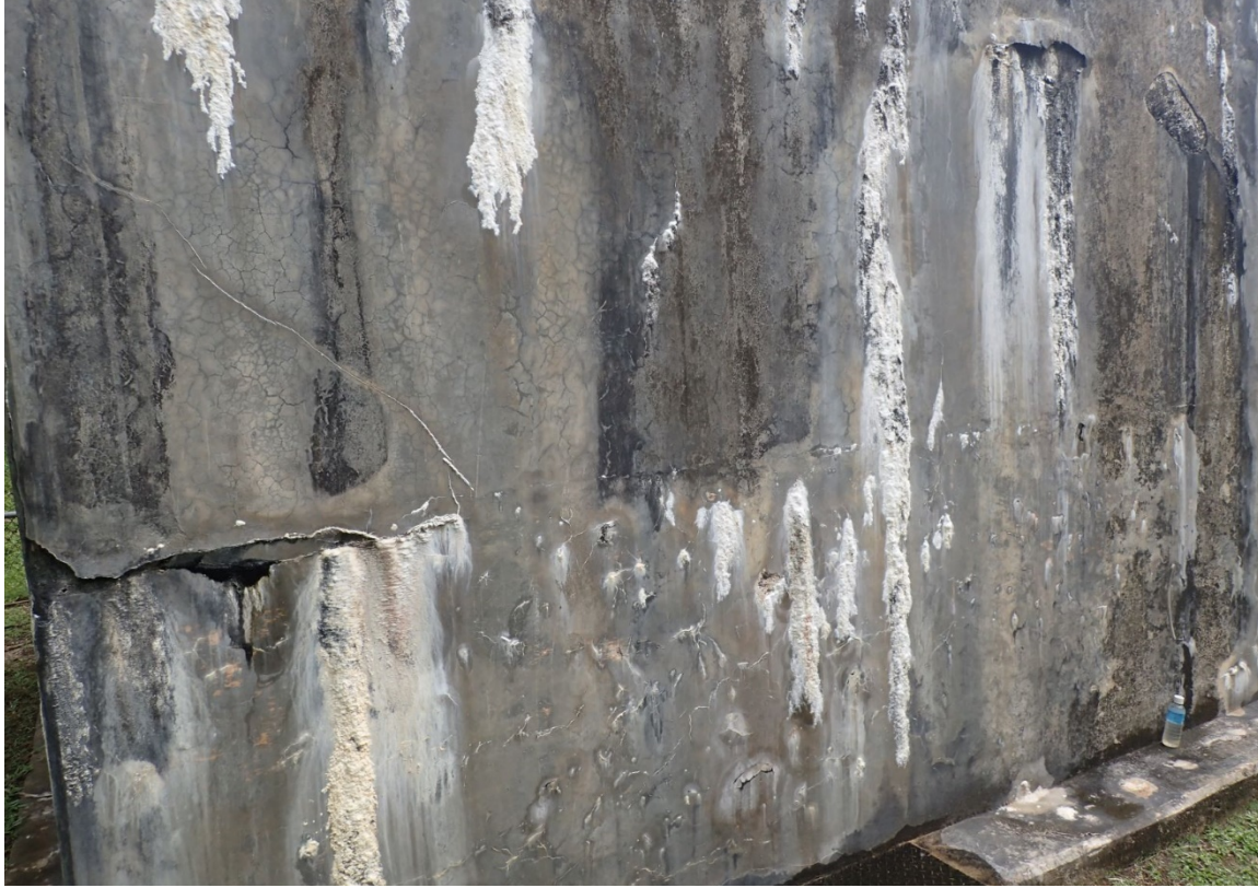
Figure 9.—Concrete efflorescence and spalling on the Ngatpang Mechebechubel clearwell tank.
