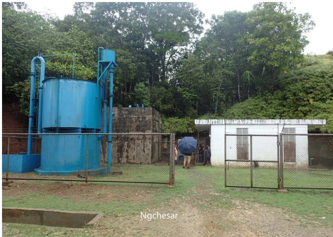
Figure 4.—The Ngchesar plant yard with (left to right) automatic valveless gravity filters, concrete chlorination storage tank (clearwell), and pump house for treated water distribution.
