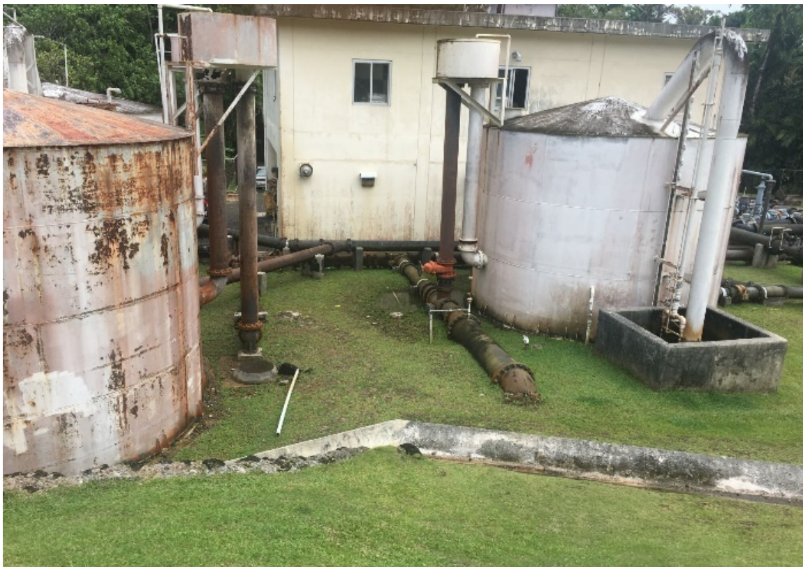
Figure 14.—The filter tanks at the Airai plant.
