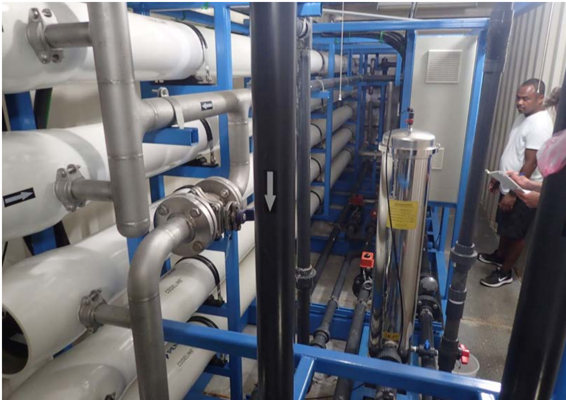
Figure 18.—The 3x2 array of 4-inch pressure vessels on the RO skid rack of the Peleliu plant.
