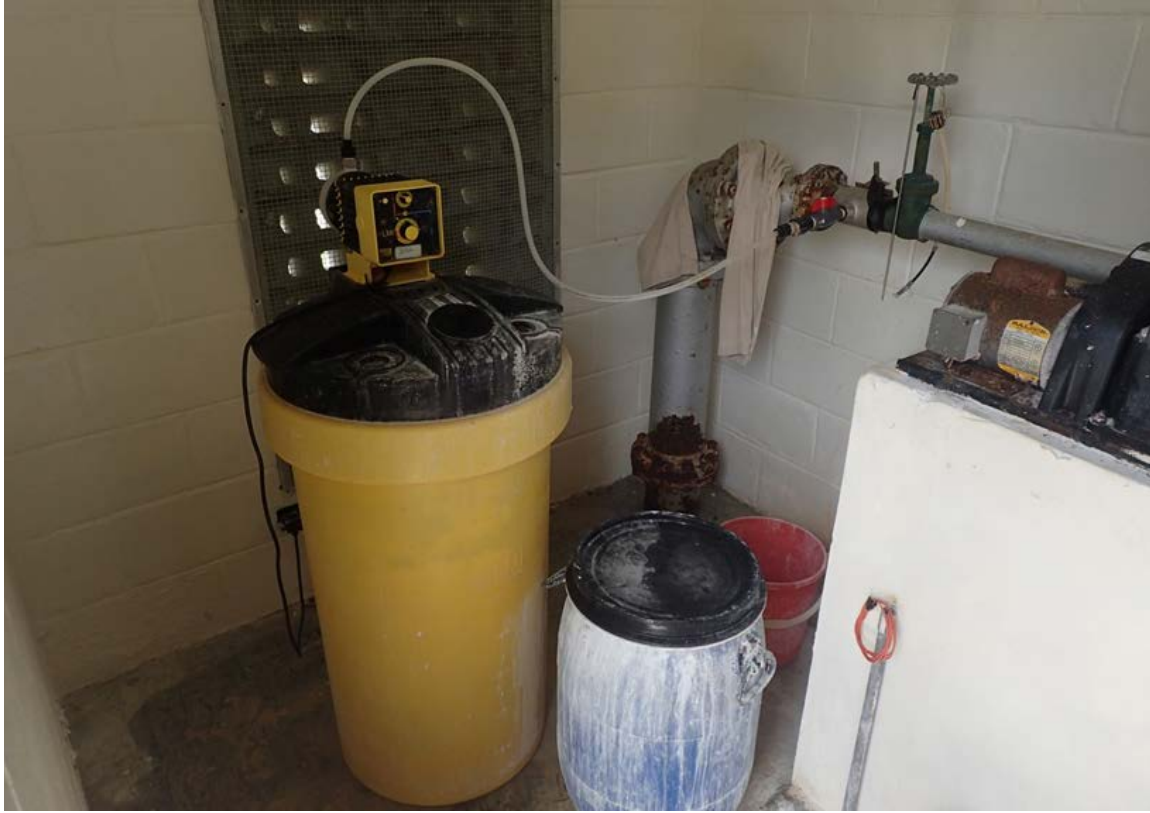
Figure 17.—The chlorine injection system for the well water that is blended with RO product water.
