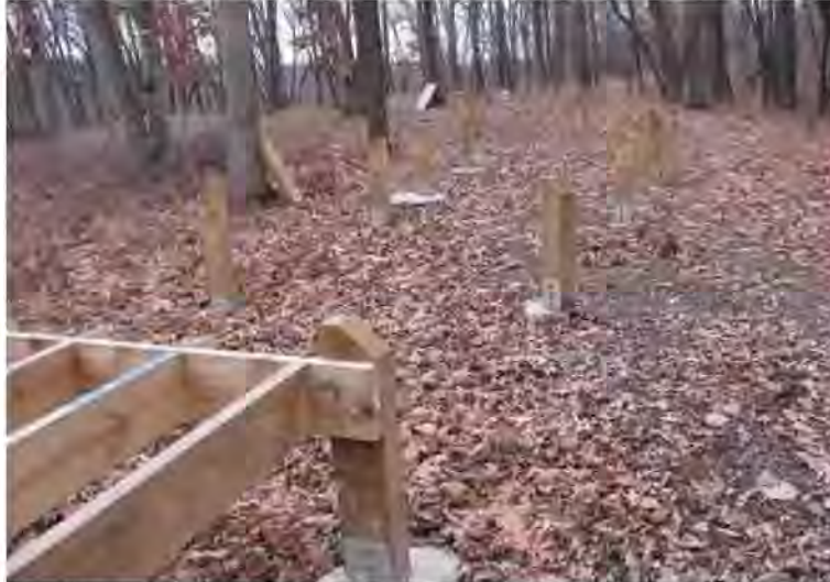
Nazekaw Terrace Boardwalk construction terminus (linear mounds visible in left background). NPS Photo.
