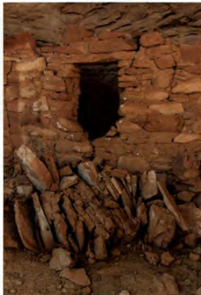
The wall of this ancient house was recently toppled.
