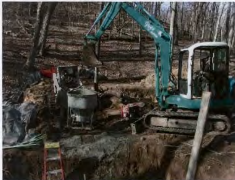
Hanging Rock Bridge under construction (2004). A simple hiking trail footbridge was replaced with a five ton vehicle bridge. A quarter-mile long access road was blazed through mature forest to accommodate construction equipment used at the site. Despite the fact that extensive ground disturbance would be taking place in an archeological park, this work was done in the absence of any NHPA, ARPA, or NEPA compliance. NPS Photo.
