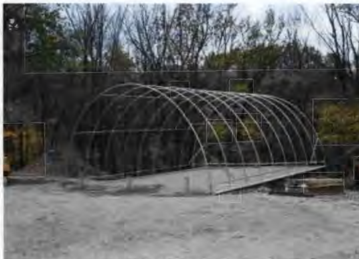
Storage shed constructed in 2007 without NHPA and NEPA compliance and without archeological clearance. Later studies revealed that it may have disturbed a remnant mound. NPS Photo.
