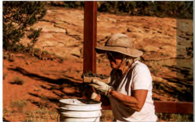
Janet Lever-Wood helps build a new information kiosk at Cave Towers. FCM thanks the Utah State Institutional Lands Trust Administration for partnering on the project.
